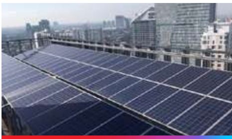
Solar Cell at Office Building
